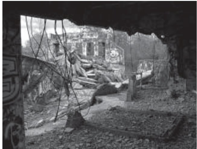
Hilltop Ward has fallen into total disuse since its days as a hospital ward and then a search and rescue training site. Though fenced in it has become a safety hazard for people cutting the fence for unauthorized access and illegal activities.
